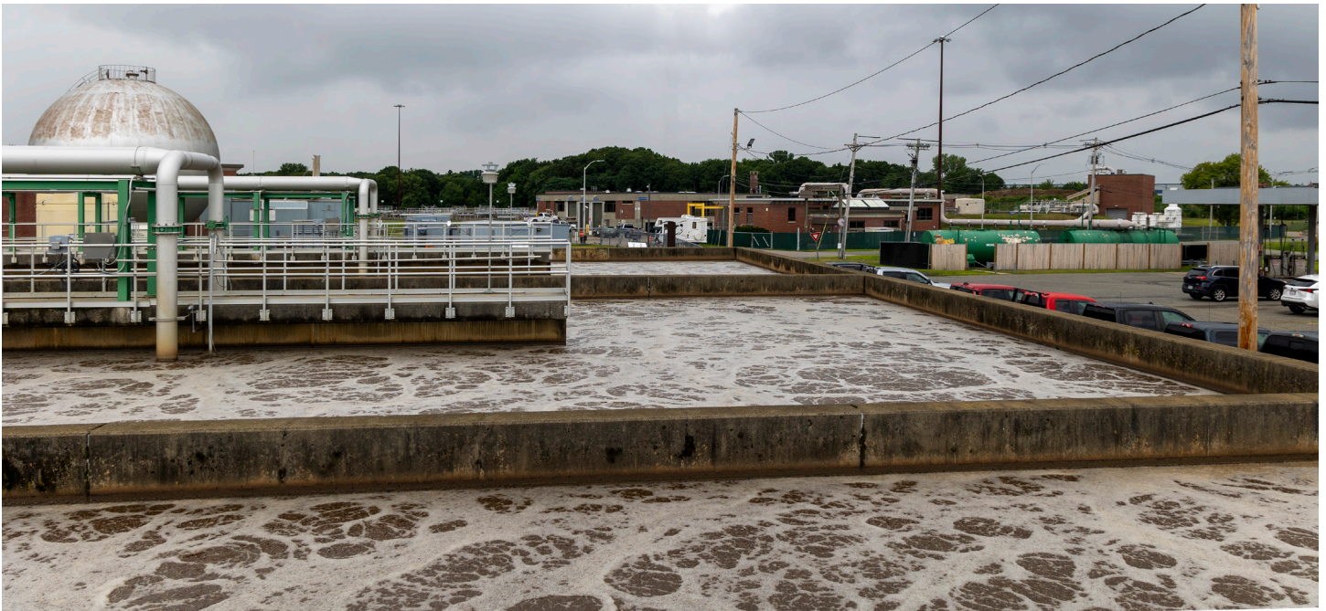
Brockton AWWRF South Aeration Basins
