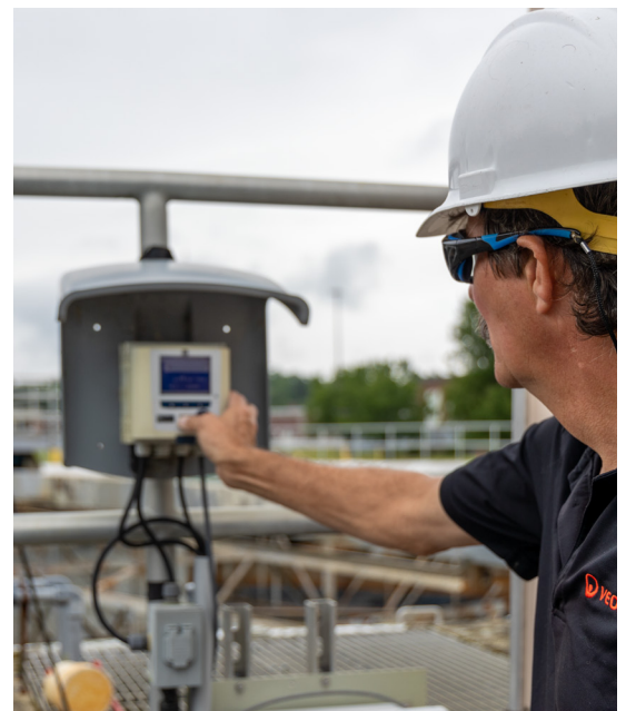
John Downey checks sensor readings on an IQ SensorNet 282 controller
